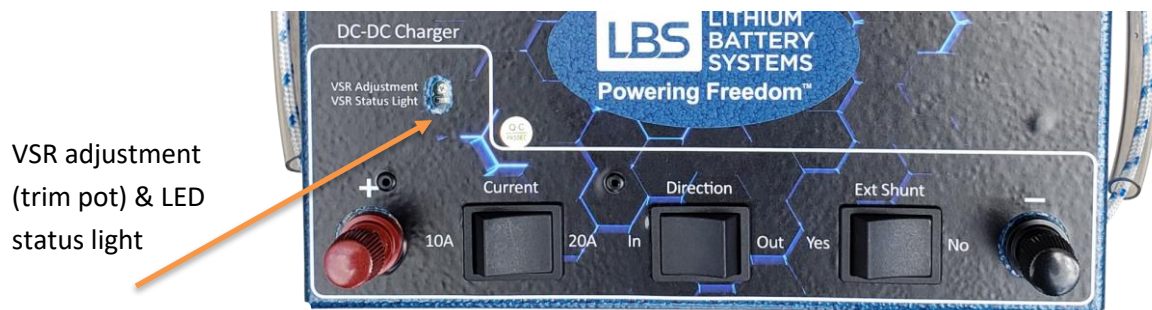
Figure 3 – DC-DC Charging Terminal Connections
